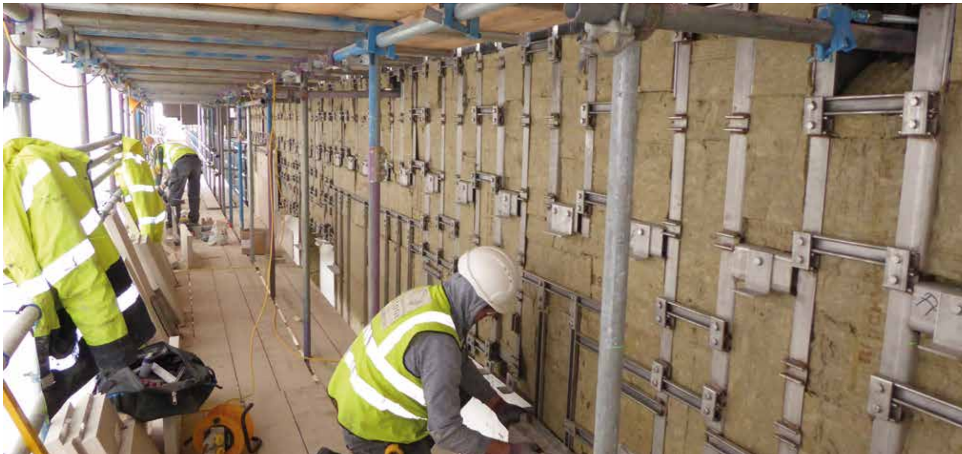
Above and below. A project at Canary Wharf where Harrison Goldman designed an exoskeleton in 6mm steel to hold the Jura limestone cladding.
